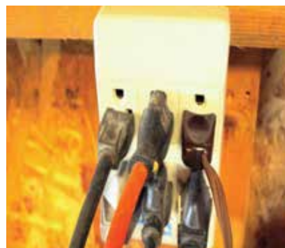
Today's increased demand for energy can overburden an older home's electrical system, like this one.
