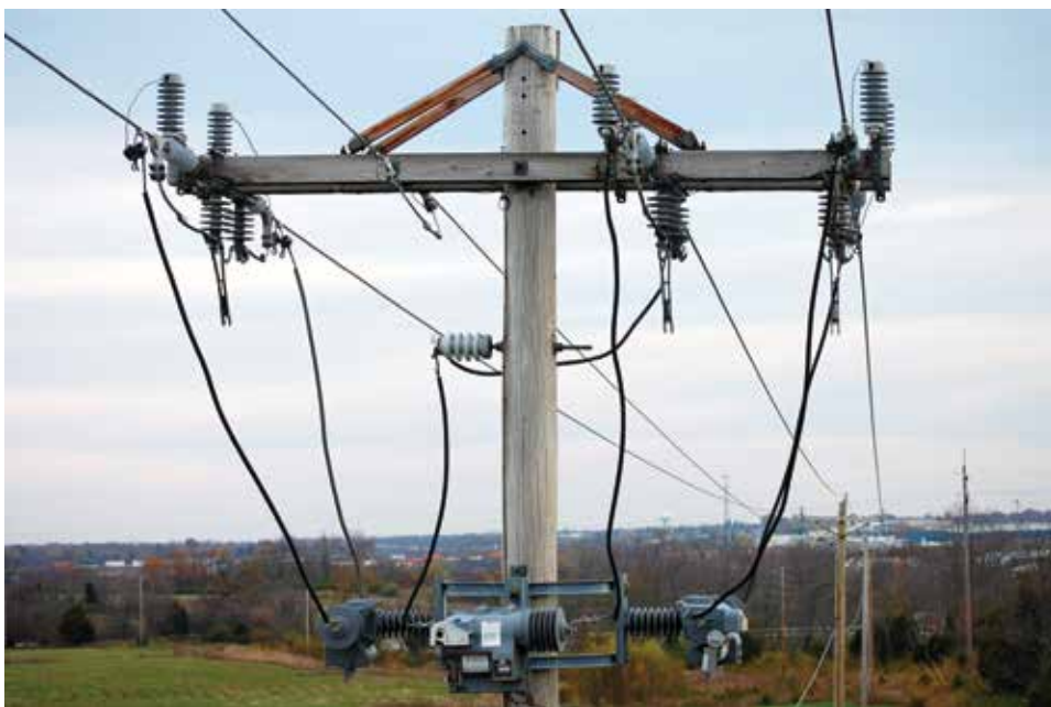
Reclosers protect lines and members from short circuits, and they allow temporary faults to clear, which helps keep service energized to the member without needless interruptions.
