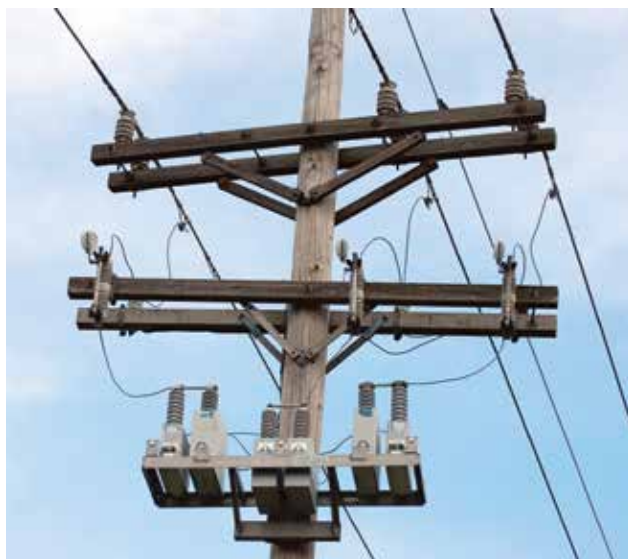
Capacitors improve the power factor on the utility lines—they prevent power from being wasted and help boost the voltage on long rural distribution lines.
