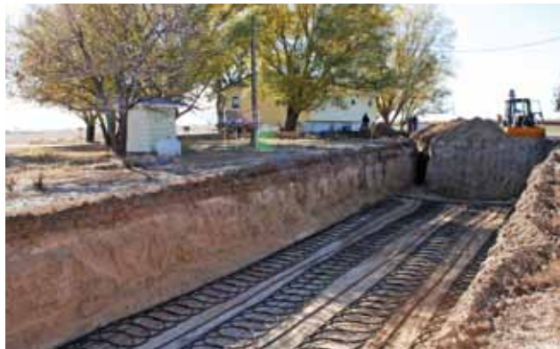
Caney Valley provides a $200 rebate for ground source heat pumps like this one.
